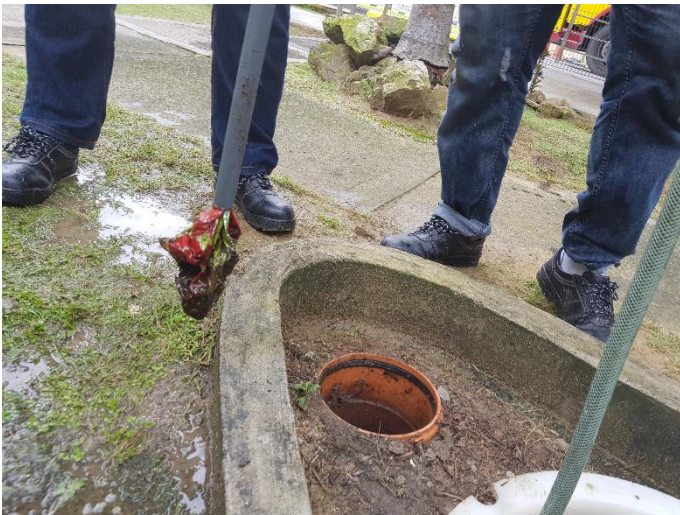
It was plastic , stone and debris found stuck at the bottom of collection sump Cleared with provided maintenance tools
