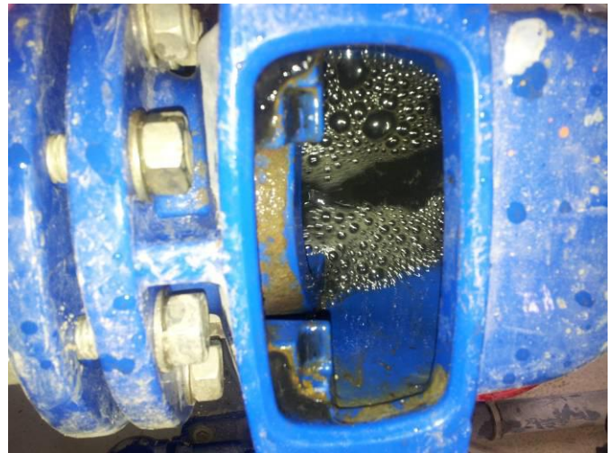
discharge pump is turned on, no water flowing
